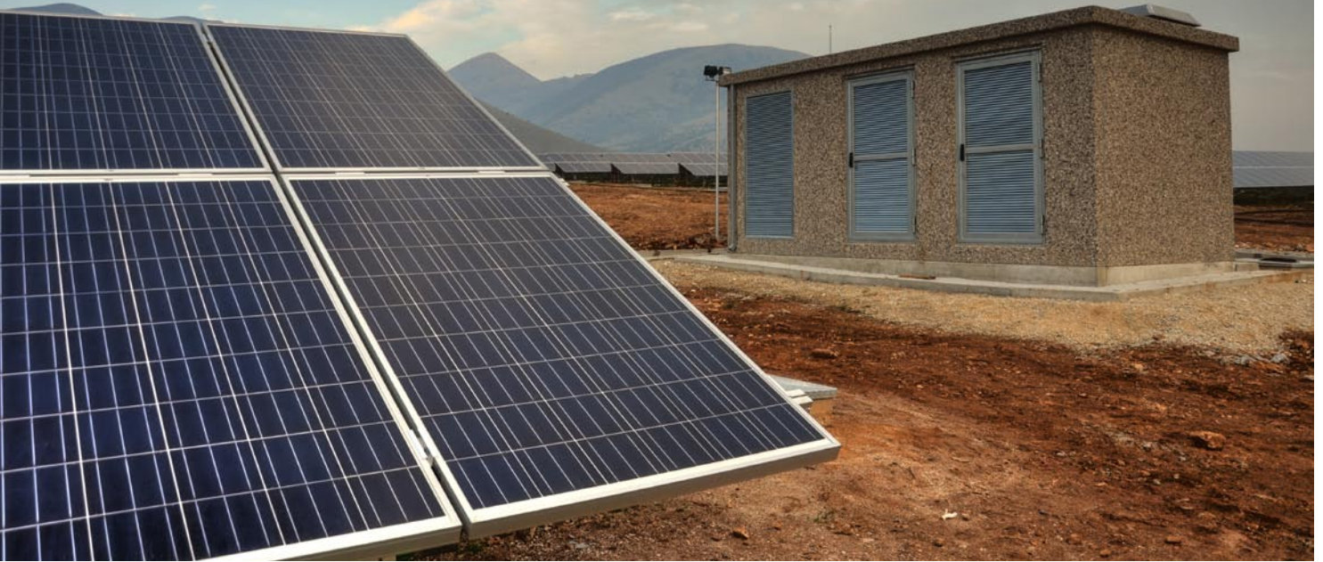
Financing larger projects may prove difficult however the rooftop market is growing.
